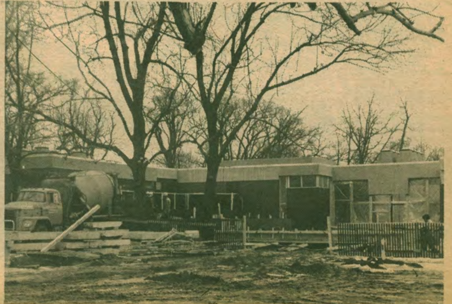
At last! The addition to our controversial new SUB is finally under construction. The darling of the Administration is expected to be completed by September and will be full of many things to amaze and delight us. Shown is a cement truck, some trees, and a long low building.
