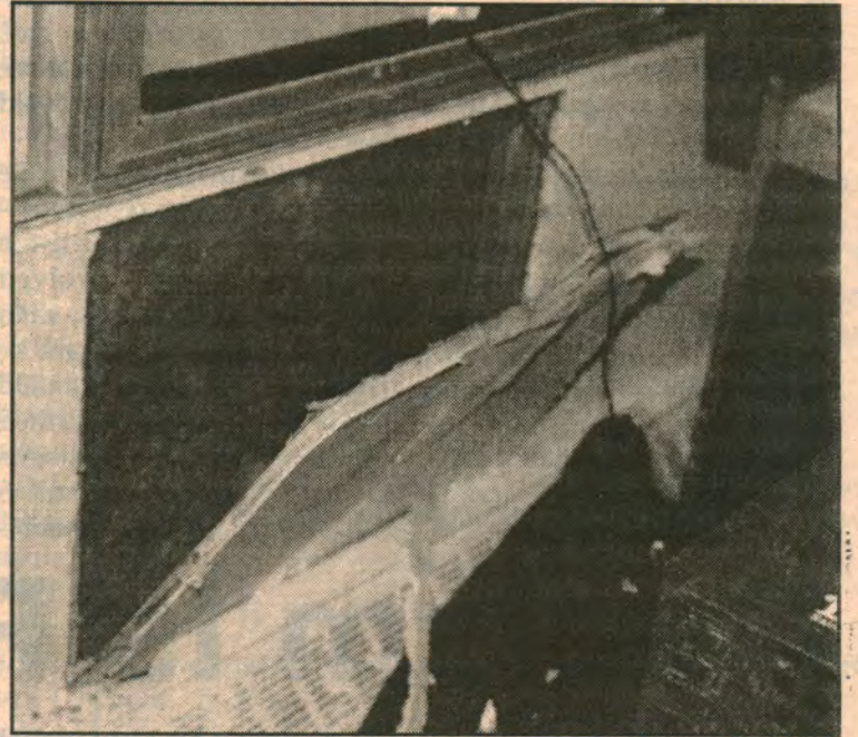
ANCHORS AWAY: A SECTION OF JASON GUIDRY'S WALL TOPPLED OVER ON THE 22ND FLOOR IN LOYOLA RESIDENCE THIS PAST DECEMBER, ALLOWING AN INFLUX OF ICY WATER INTO HIS ROOM. GUIDRY SAYS THAT THE WHOLE FLOOR IS IN NEED OF REPAIRS.
