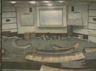
THE CONFERENCE ROOM IS STILL UNDER CONSTRUCTION, BUT OFFICIALS SAY THE DOORS WILL BE OPENED SOON.
