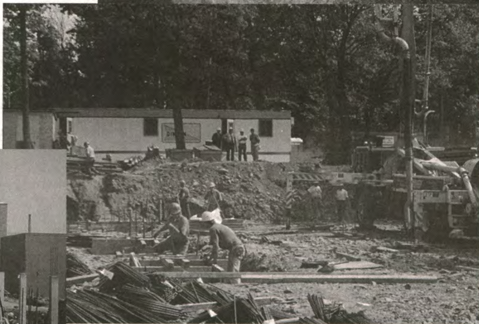
Construction workers are working all day to ensure that the new school will be completed by September, 1998.
