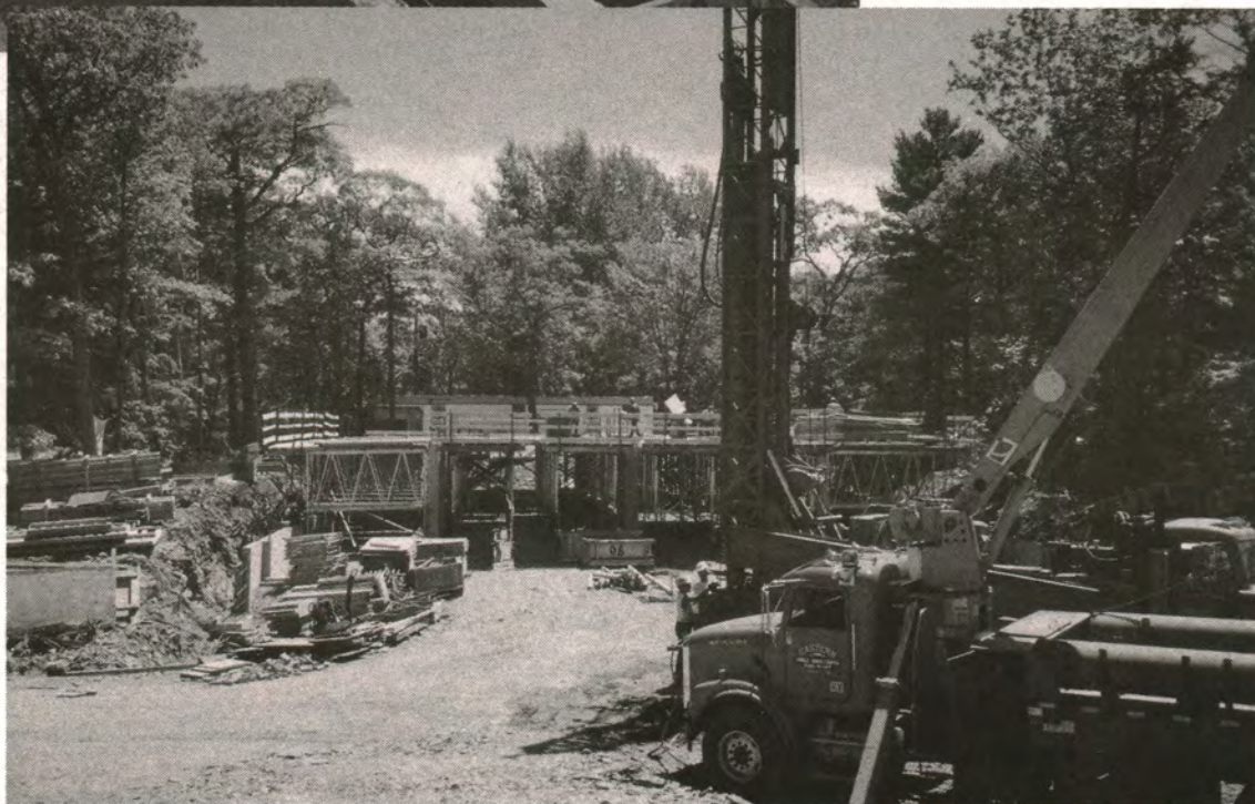
The new school begins to take shape at the end of July.
