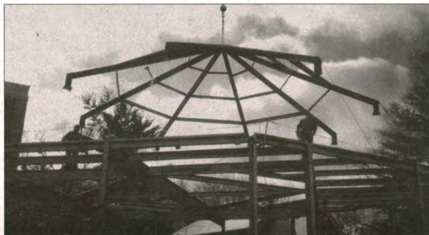
The triangle shaped steel is lowered on the roof of the large lecture hall of the new school on November 28.
