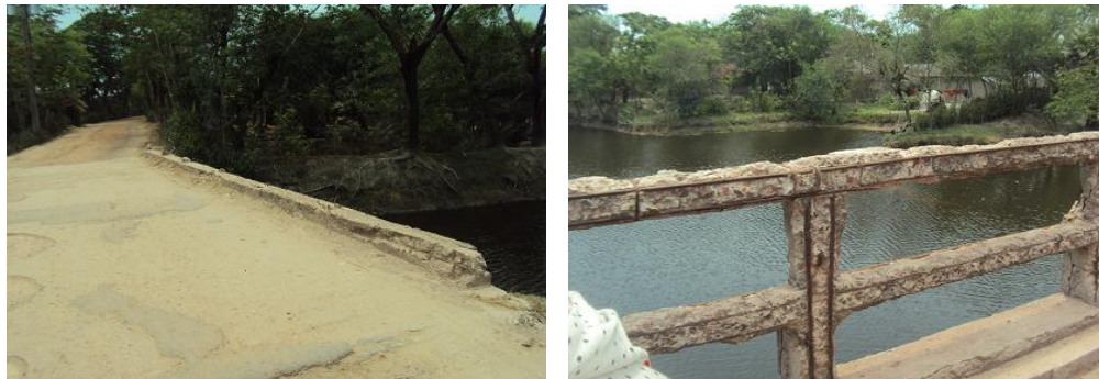
Pictures 1.13: One side of the railing of the bridge has been disappeared, and another side is also damaged due to cyclone 'Aila' that occurred in 2009. Source: Author's photograph.
