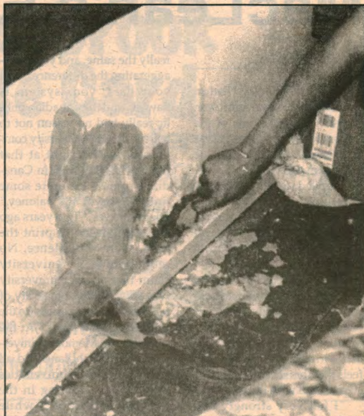
SOME OF THE DESTRUCTION CAUSED BY WATER LEAKAGE FROM THE ROOF OF THE LOYOLA RESIDENCE
