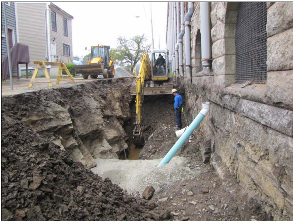
PLATE 11: Excavation of trench adjacent to bedrock ledge along south side of building. Facing west.
