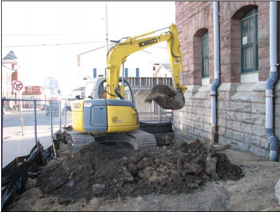
PLATE 6: Initiation of excavation at the northeast corner of the Armoury. Facing east.
