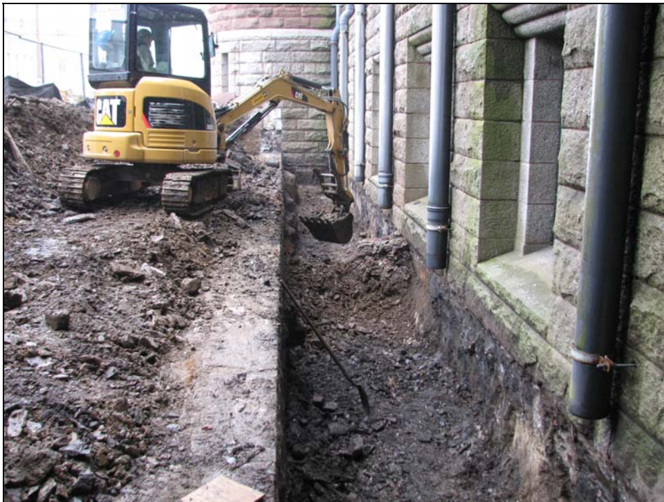
PLATE 7: Excavation adjacent to retaining wall along north side of building. Facing east.
