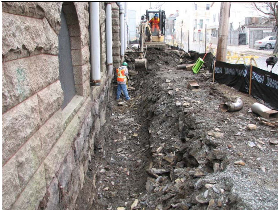
PLATE 9: Excavation of trench adjacent to bedrock ledge along east side of building. Facing north.
