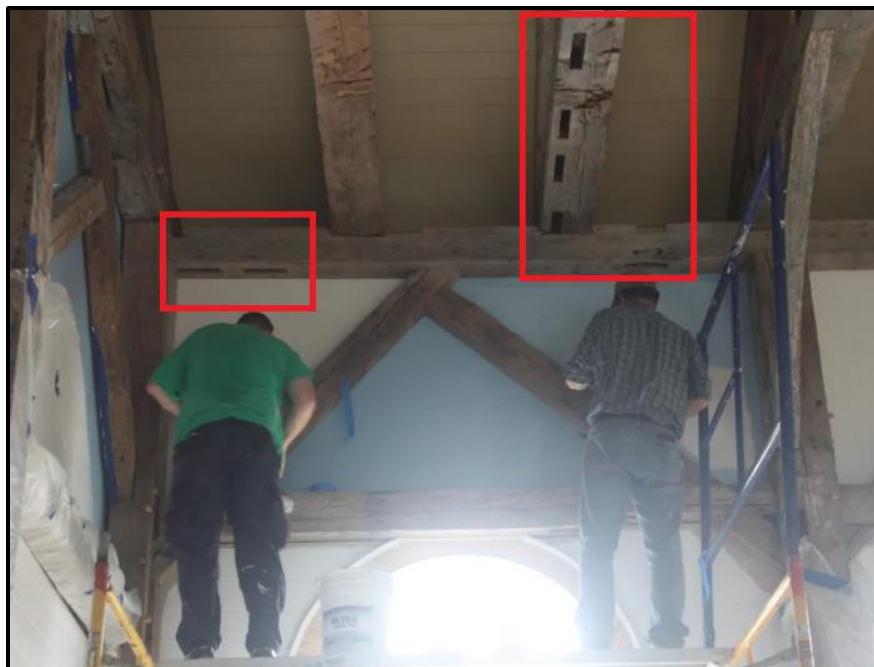
Figure 11: Mortise Joint holes visible in areas outlined in red. Joints of the structure beams that do not have a purpose in this structure. Photo taken in 2015, during buildings reconstruction in Louisiana. Rhodes 2015
