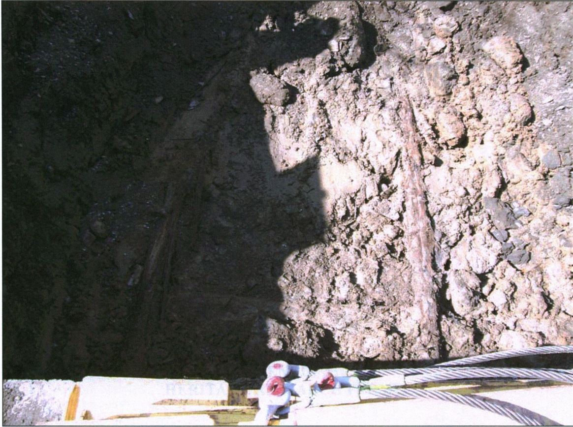
Plate 5: Wooden cribwork of a wharf approximately 1.8 metres below the asphalt surface, facing west.
