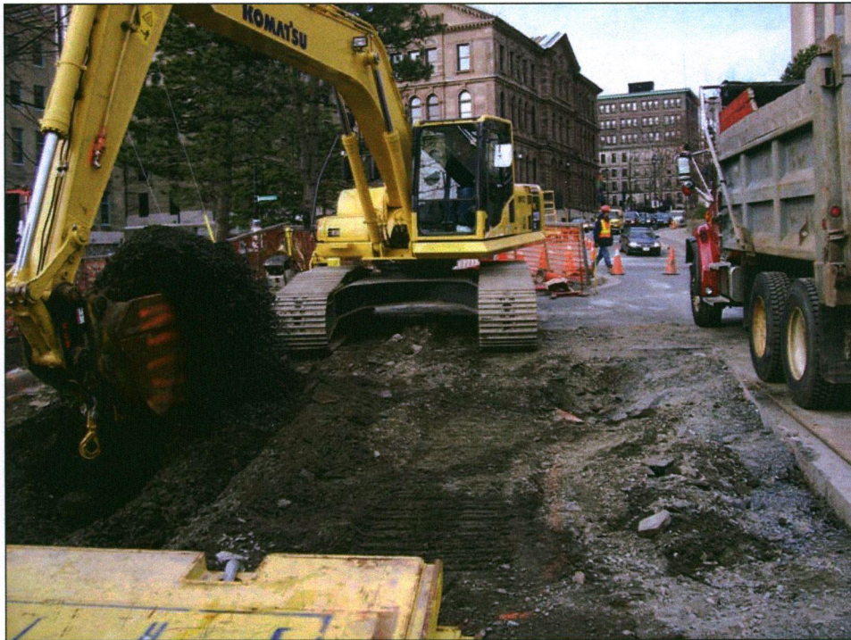
Plate 1: Excavation area on the west side of the Nova Scotian Crystal building for the installation of a pumping station, looking up George Street.
