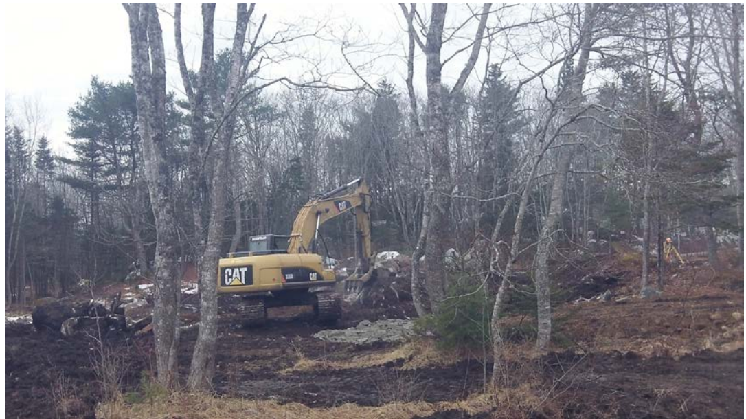
Monitoring building site ground disturbance and clearing. Some remnants of snow in the background. (K. Cottreau-Robins, March 2014)
