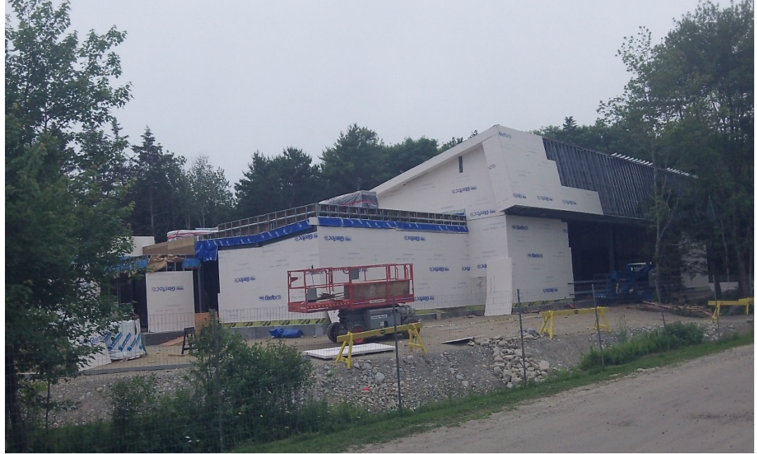
Checking in on the building site following the monitoring stage. (K. Cottreau-Robins, July 2014)
