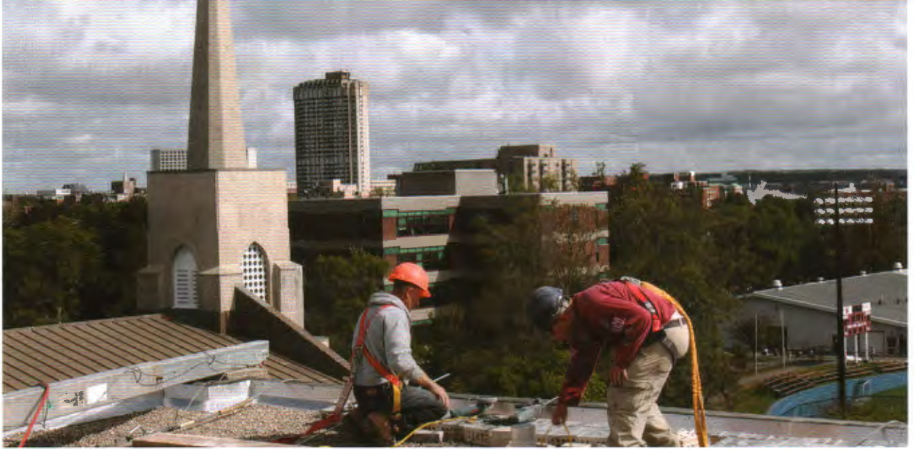
Workers replacing the roof of the McNally Building had a spectacular view of Halifax. photo: Paul Darrow
