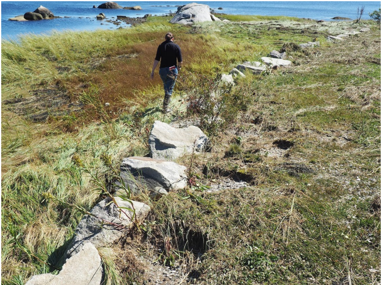
Figure 9: A portion of the park's low retaining wall, looking south from the eastern side of the park at very low tide. This photo was taken the day after the site was hit by Hurricane Lee in September 2023; at center foreground is some of the erosional damage caused by storm surge. A brief pedestrian survey following the storm did not reveal any exposed artefacts or remains from these washed-out areas.
