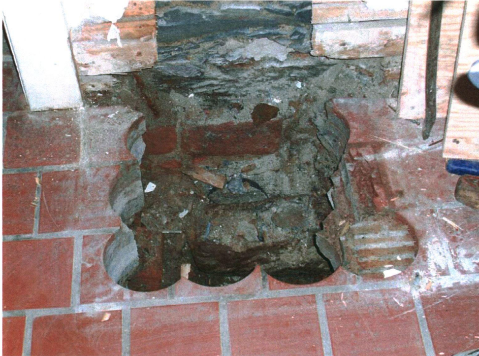
Plate 5: Stone and brick footing or threshold beneath the existing floor on the north side of the kitchen.
