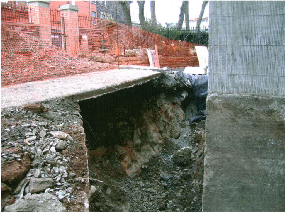
Plate 9: South side of Government House near southeast corner showing previous disturbance and modern fill associated with sanitary sewer service.
