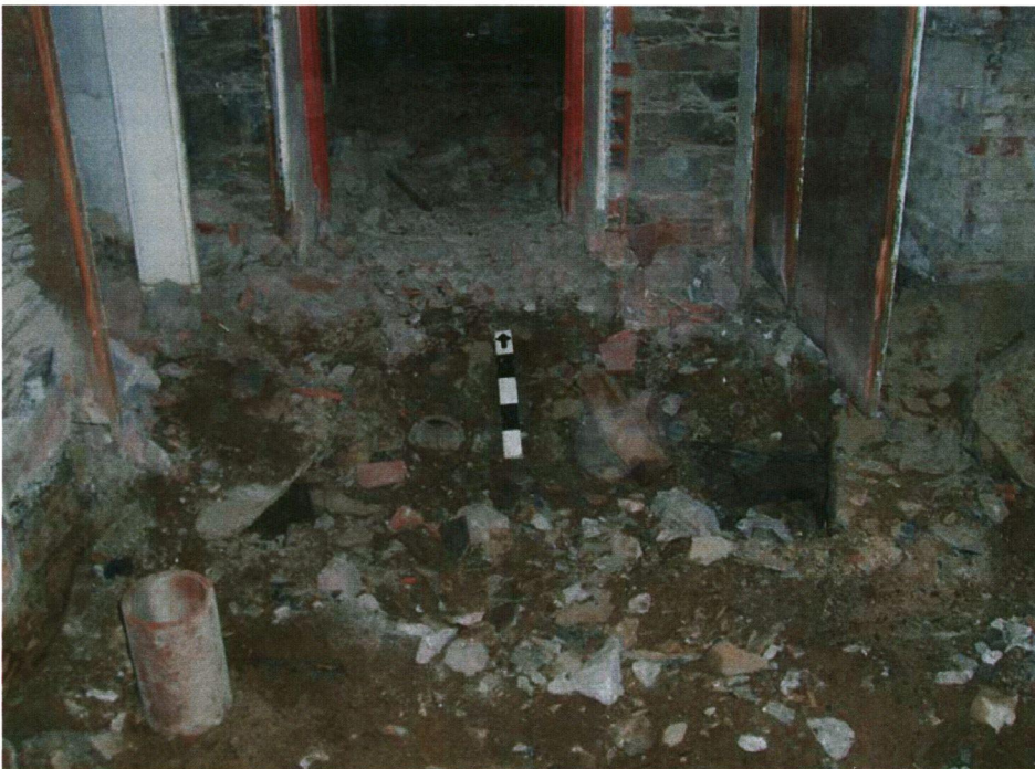
Plate 12: Stone-lined drain running east-west through the storage room (horizontal in photo), and intersecting north-south drain at course earthenware pipe junction, looking north.
