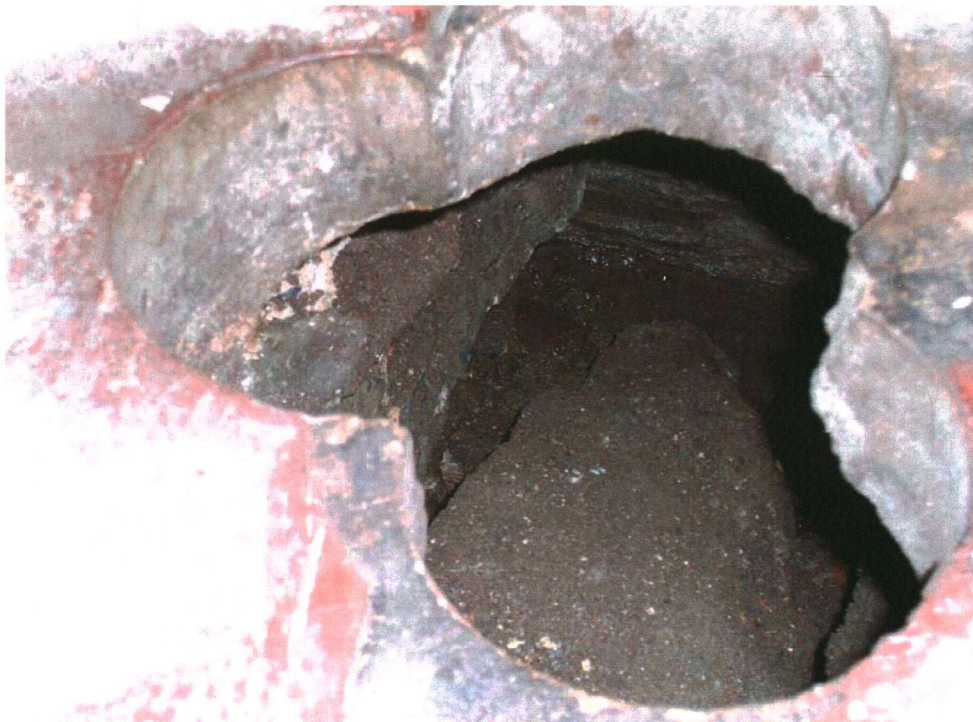
Plate 6: Stone drainage feature beneath the existing floor, east of the locker room.
