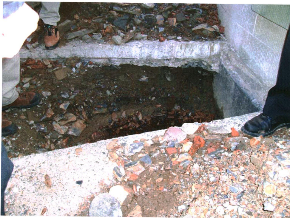
Plate 2: Removal of concrete and fill from north end of moat for initial inspection on 21 November 2006.
