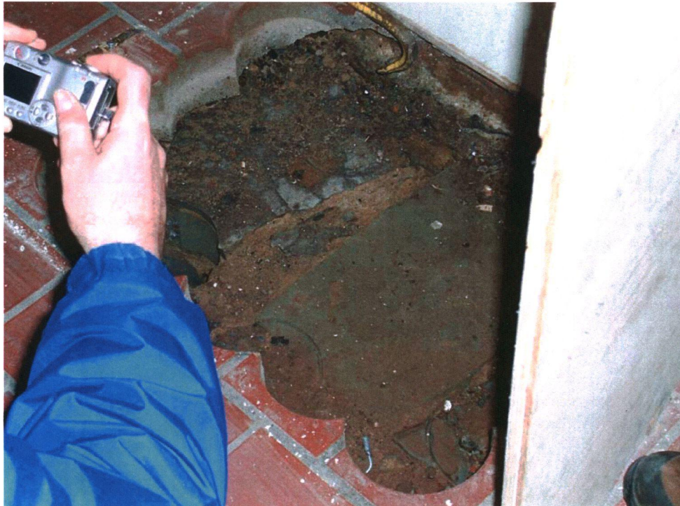
Plate 7: Slate floor tiles beneath the existing floor on the north wall of the locker room.
