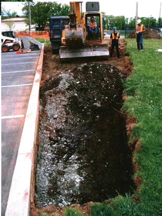
Plate 2: Modern gravel fill under concrete curb at north edge of access road, looking east.
