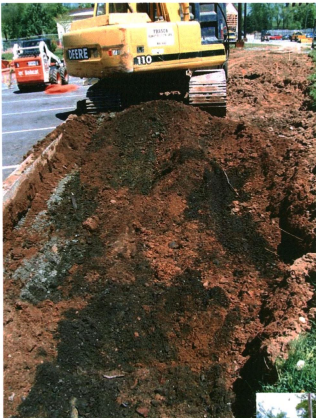
Plate 1: Redeposited refuse materials (dark soil matrix) excavated during construction of the access road from Summer Street north of the Wanderer's Grounds, looking east.
