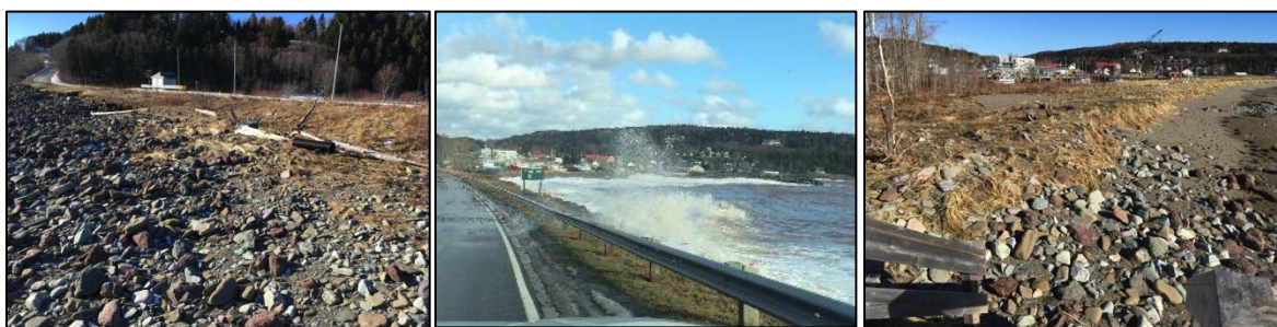
Figure 4.5. Gale-force winds on December 30, 2016 caused large waves that further damaged the Alma Beach revetment. Boulders from the revetment have been pushed beyond the beach access stairs (Jan. 2017). (centre photo courtesy of Robin Stuart, 2016)
