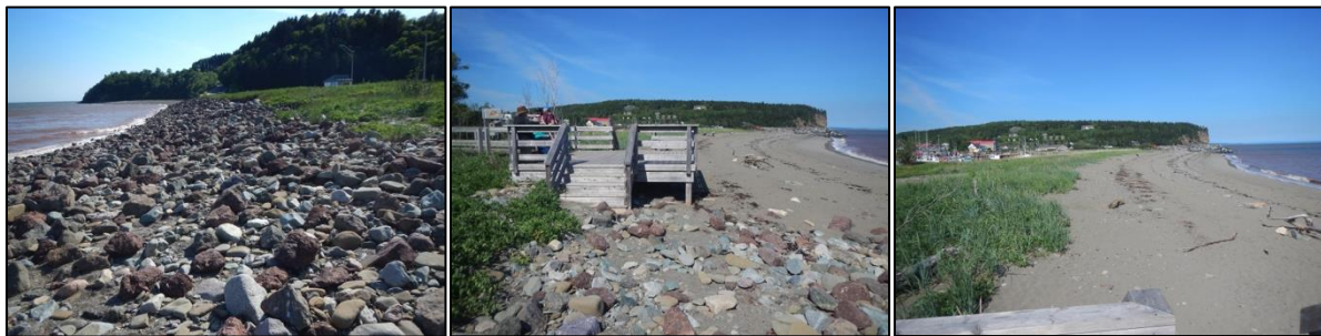
Figure 4.4. Alma Beach access stairs on June 27, 2016 and extent of boulders from the damaged revetment at the time
