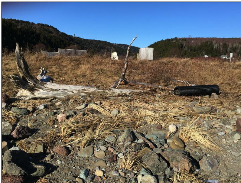
Figure 5.1. Resting place of a pipe washed out of the Alma beach revetment in a storm on December 30, 2016 (Jan. 2, 2017)
