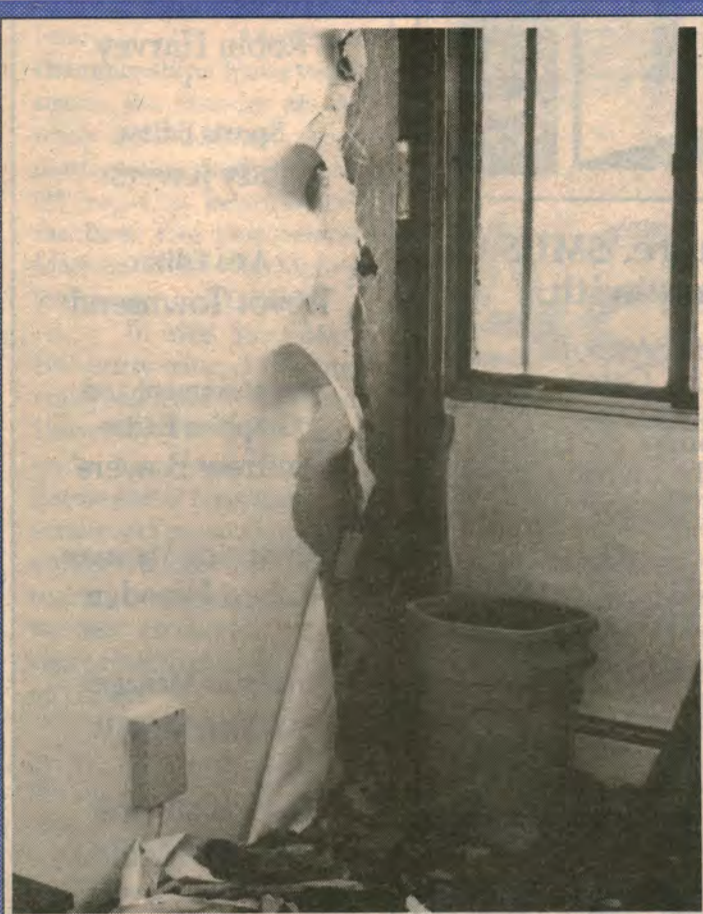
Residence students were treated to broken water pipes, exploding walls and flooded rooms last week in Loyola.
