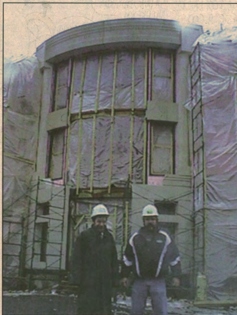
ABOVE: PAUL DIXON, DEAN OF COMMERCE, AND LEONARD DYKENS, CONSTRUCTION SITE MANAGER, STAND IN FRONT OF THE SOBEYS BUILDING. RIGHT: ONE OF THE NEW CLASSROOMS LOCATED ON THE GROUND FLOOR. BELOW: LOOKING UP FROM THE MAIN ENTRY TO THE SKYLIGHT ABOVE THE NEW LOFT STYLE BOARDROOM.
