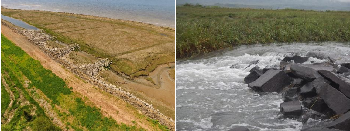
Figure 52: Rock aprons implemented across the borrow pit at RD_01 (right). Ebb tide moving over the rock aprons in RD_01 (left).
