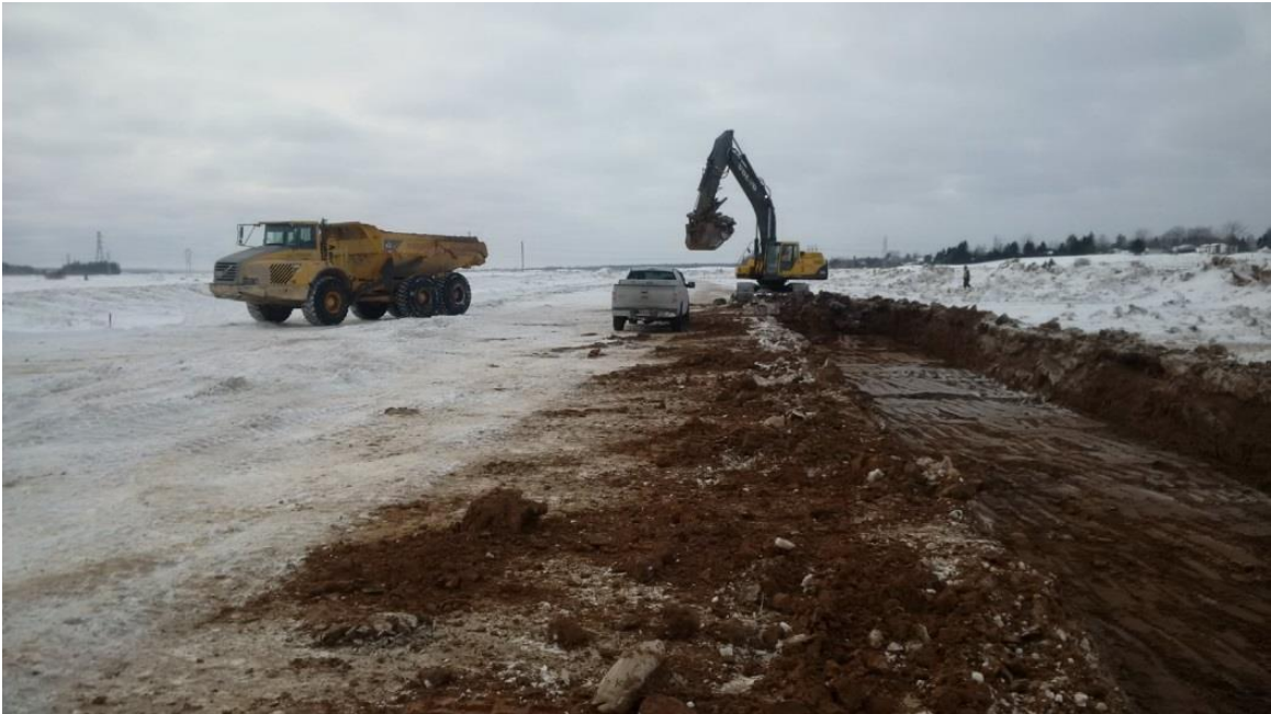
Figure 26: Borrow pit excavation using a long-reach excavator. Photo credit - Carl Esau, NSDA, winter 2015.
