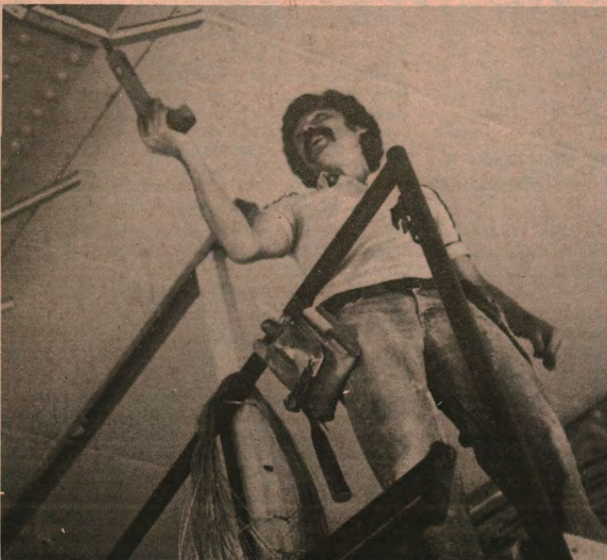
Renovations to the Theatre Auditorium started early in June, and the work is expected to be completed by September 30. Mike Gurdic, of Yorkdale Drywall, is shown installing the acoustic ceiling.
