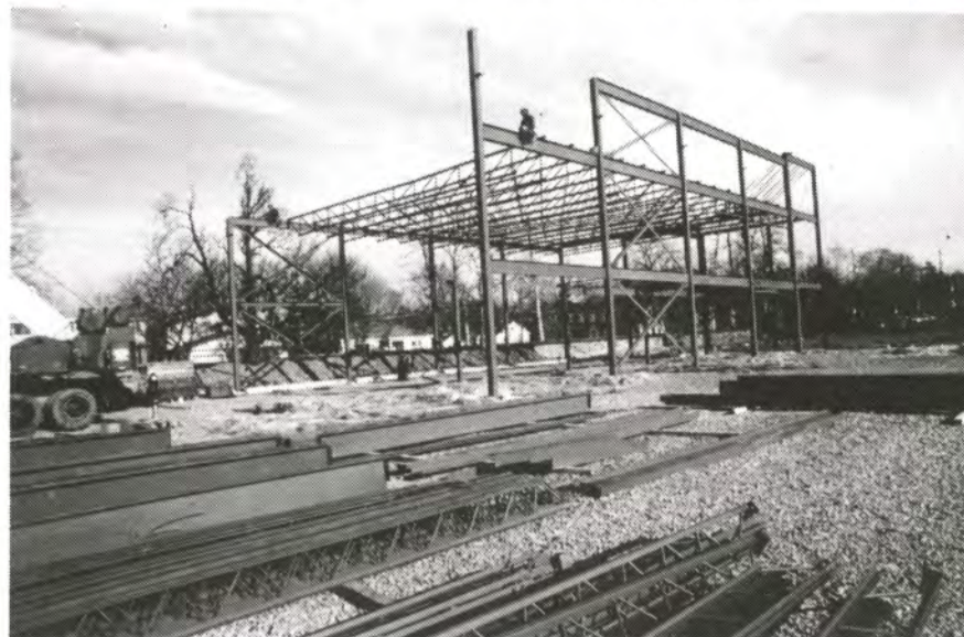
The steel construction on the new Fitness and Recreation Centre is proceeding so quickly that this photo will be out of date by press time. The warm weather has seen a flurry of activity on the construction site between Huskies Stadium and Tower Road. (Chislett photo)
