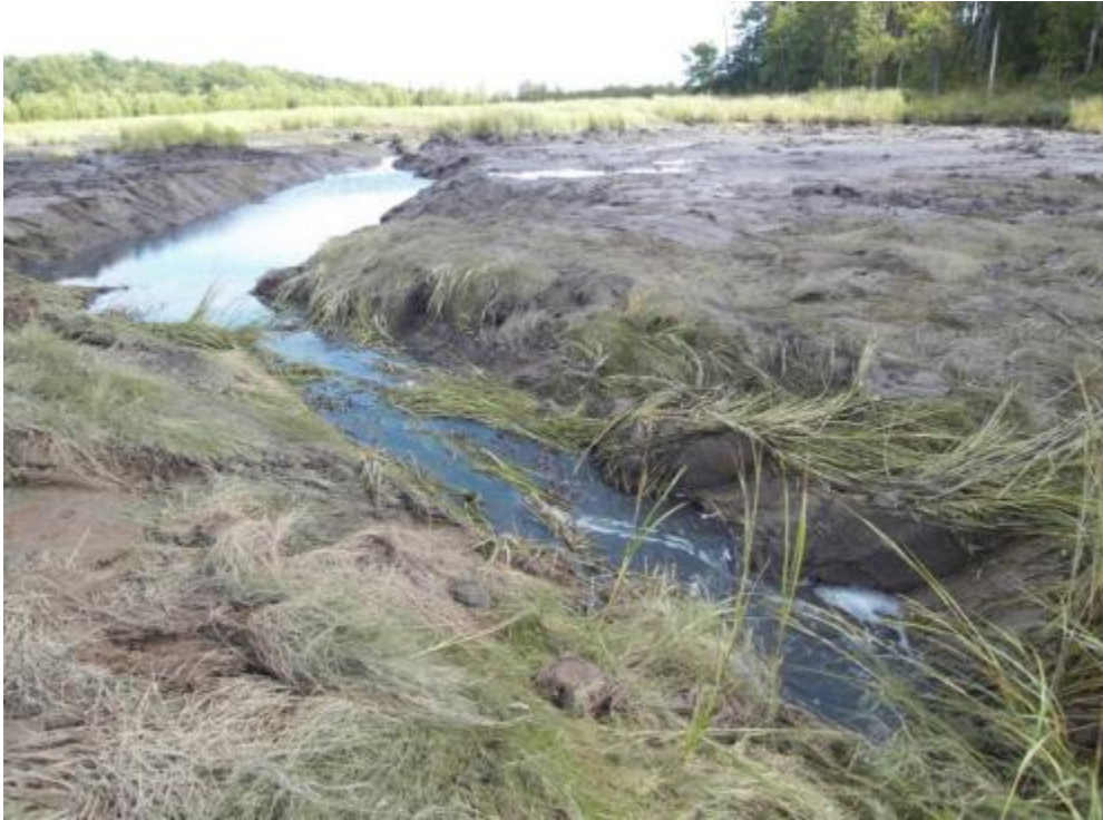
Figure 1.4. An image showing the channel construction at the Cogmagun River Restoration site following the completion of the construction work. Photograph by J. Graham, 23 September 2009.
