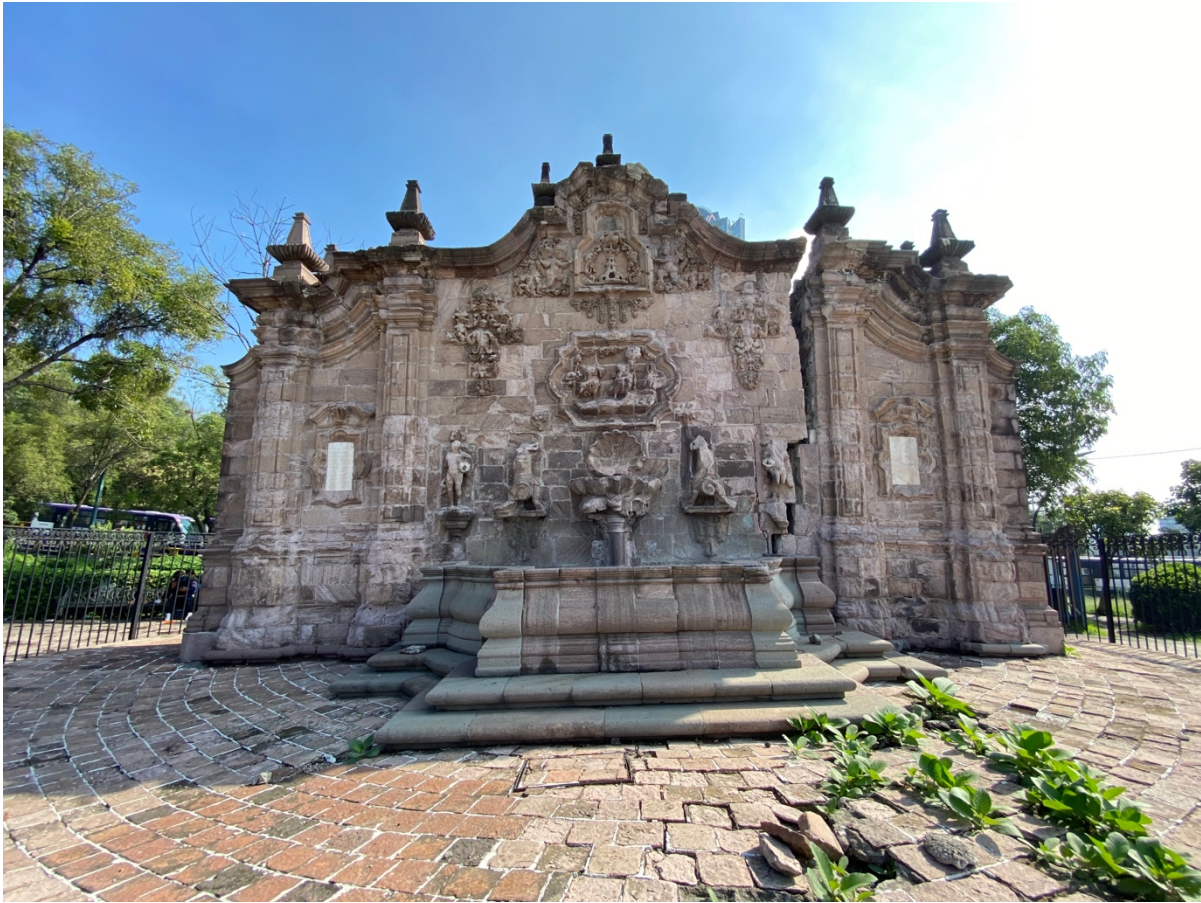
Belén Fountain. The Mexico City subway passes right under it, and as a result the fountain now presents a big crack on the right. Historians and conservators have demanded the government make efforts to preserve the fountain properly, to no avail. Photograph by Víctor Fuentes, 02 September 2023.
