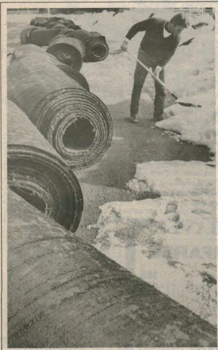
Dateline SMU - March 25- removal of old turf and underpad by Balsom Corporation of Missouri. May 1- Astroturf arrives from Georgia and gets laid down June 1- Huskies Stadium renovations complete.
