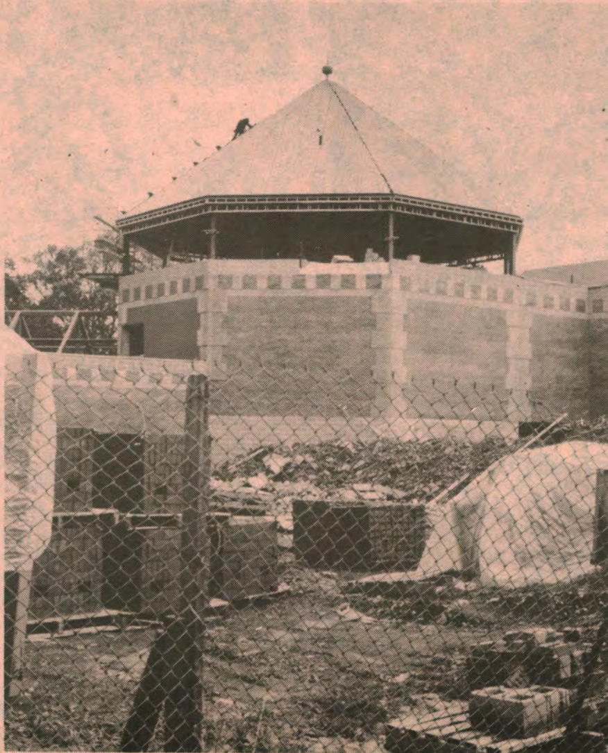
Elegant brickwork supports the cupola that will house the main machinery for the Fitness and Recreation Centre
