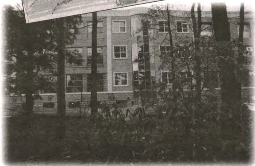
Top: architects drawing of the courtyard entrance to the Sobeby Building. Bottom: back view of the building as it takes shape.
