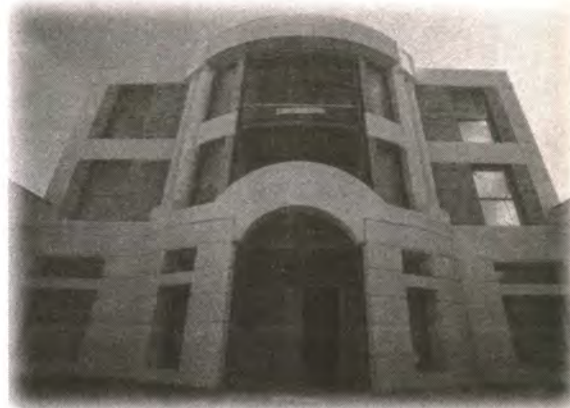
Under construction: the front of the new Sobeby Building as it nears completion.
