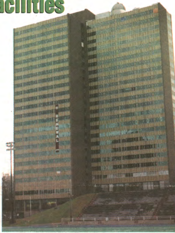
The Loyola residence is part of a $25-million dollar infrastructure renovation and renewal project in preparation for Saint Mary's bicentennial. As construction crews complete the replacement of Loyola's cladding and installation of new windows the entire interior of the residence is being renovated. The proposed renovations of Huskies Stadium, visible in the foreground, would be another extension of the renewal of Saint Mary's.
