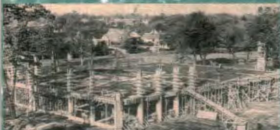
The Burke Education Centre being built in 1965 – the first free-standing library at Saint Mary's.
