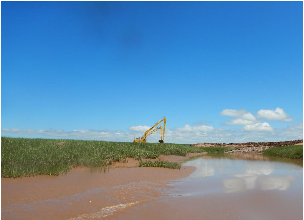
Figure 2.3: Excavation of the Windsor marsh on June 22 nd , 2020. Photo used with permission from Lachlan Rihel of the Confederacy of Mainland Mi'Kmaq (Appendix A).
