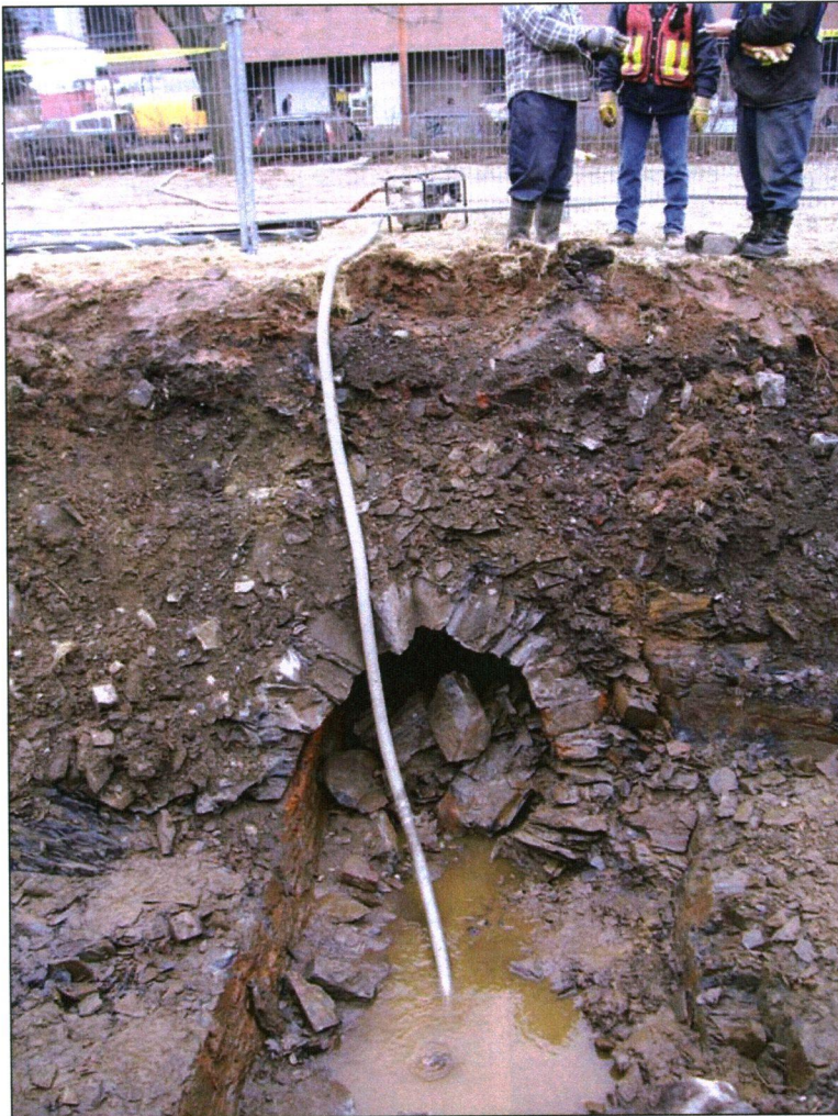
Plate 4: Mortared stone culvert in profile after removal of the top portion, looking south. On the left side of the culvert is bedrock which has been excavated.
