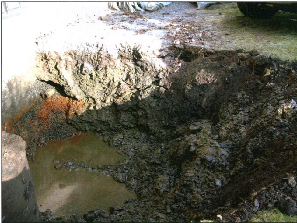
Plate 5: Disturbance adjacent to the museum building as a result of previous catch basin installation (catch basin can be seen in the left foreground).
