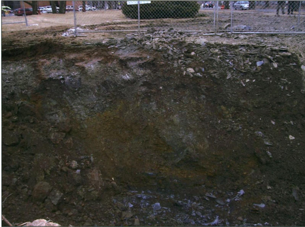
Plate 1: Disturbance on the west side of Bell Road in the area of the catch basin installation.
