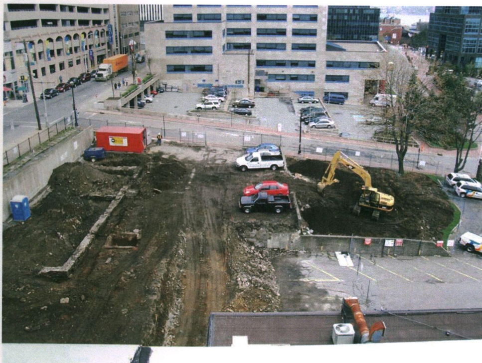
PLATE 3: Mechanical stripping of the west side of the study area showing the tops of archaeological features along Hollis Street.
