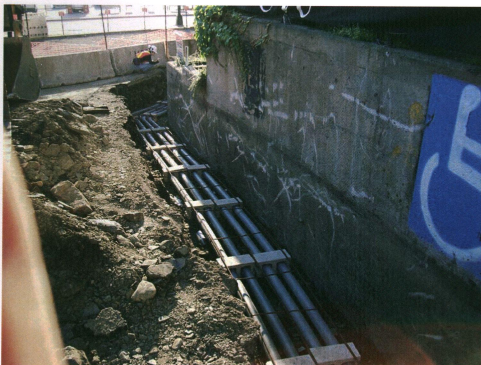
PLATE 4: Excavation of the conduit trench on the north side of the Brewery building.
