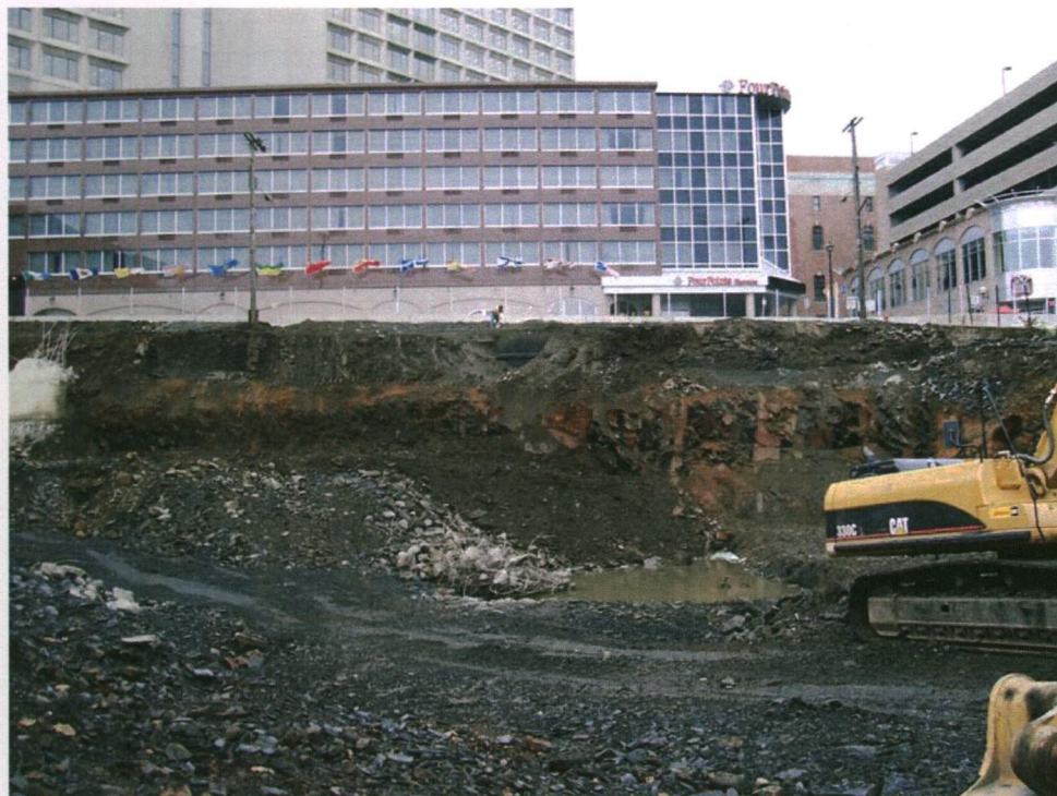
PLATE 5: West side of the study area along Hollis Street after removal of the concrete retaining wall.
