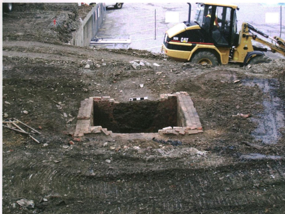
PLATE 6: Feature 1 showing previous disturbance to the east wall of the structure, looking east.
