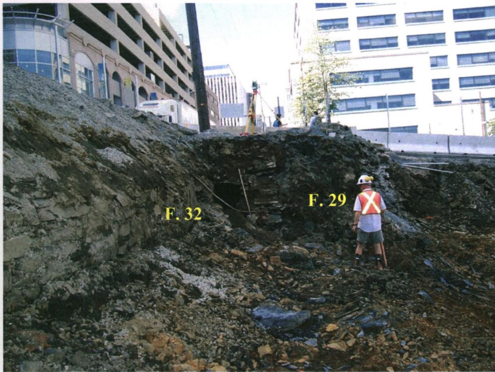
PLATE 19: Features 29 and 32 behind concrete retaining wall and fill on Hollis Street, looking north.
