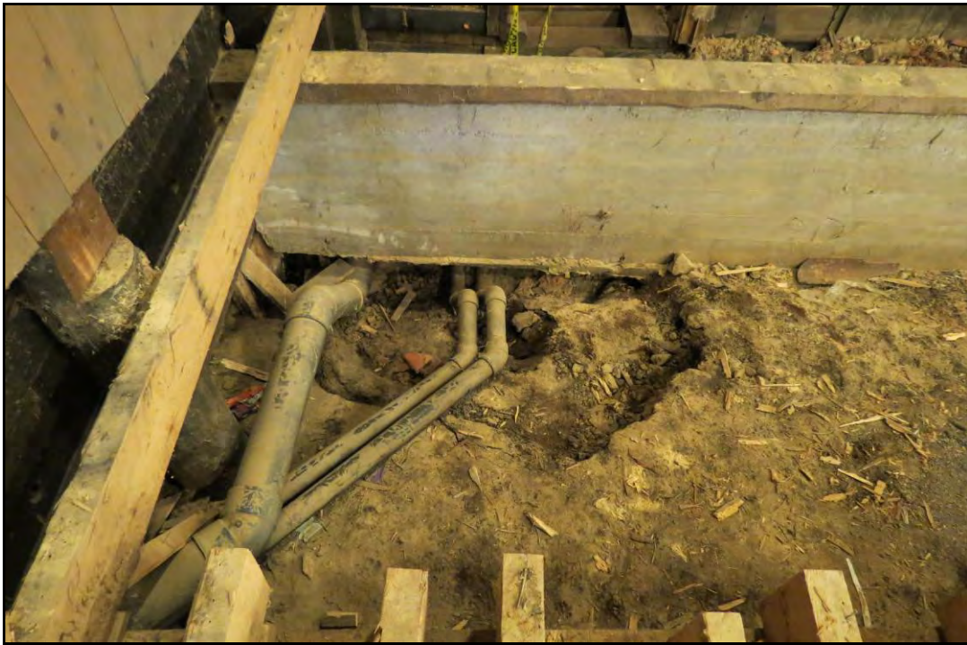
PLATE 7: Plumbing running beneath a concrete joist; October 22, 2013.
