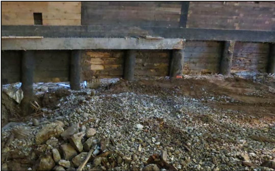
PLATE 6: Support pilings along the west side of the Inshore Fisheries Display Building; facing west; November 6, 2013.
