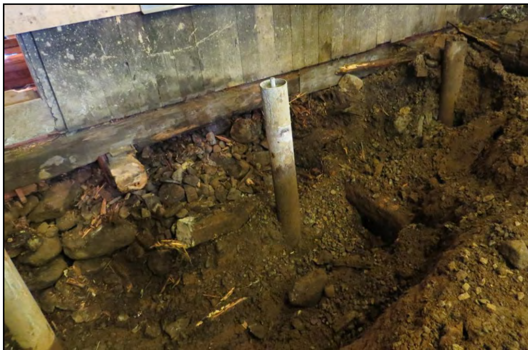
PLATE 18: Cobble fill and timber framing along south wall of the Inshore Fisheries Display Building; facing south; February 6, 2014.
