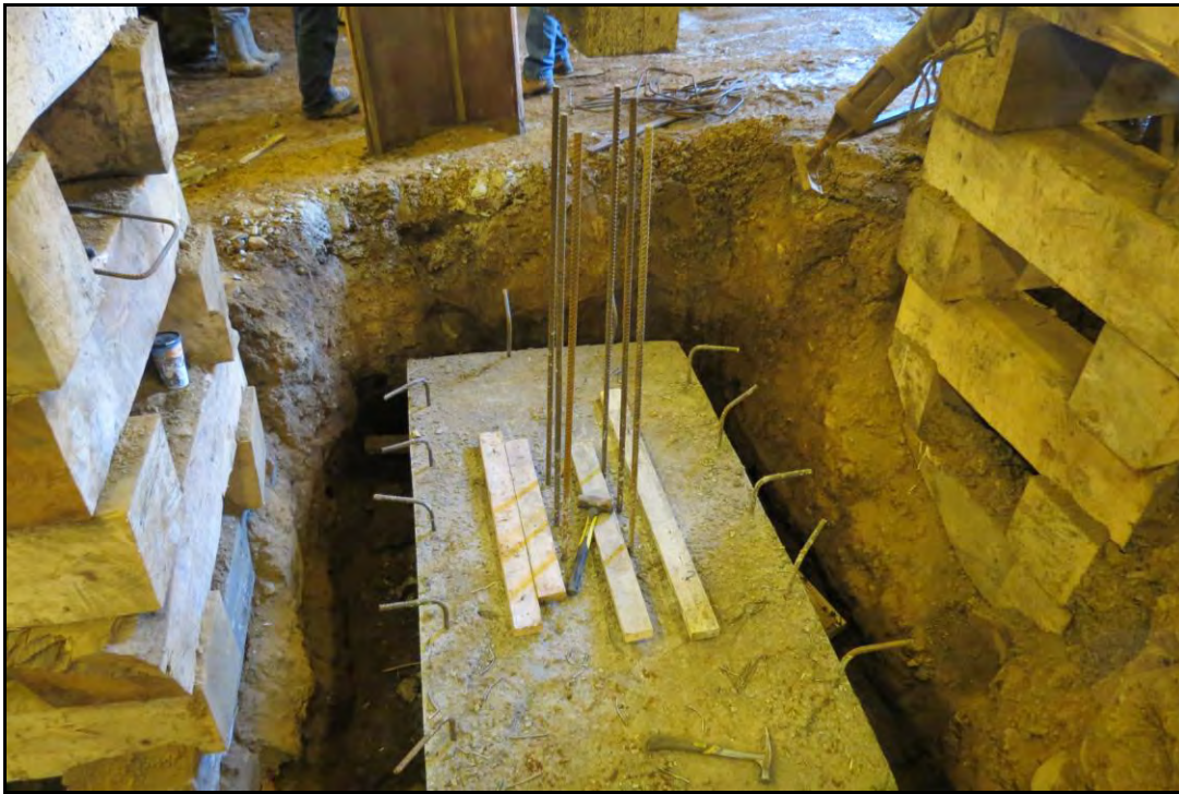
PLATE 17: Concrete piling cap set in pit dug in fill within the Inshore Fisheries Display Building; facing west; January 8, 2014.
