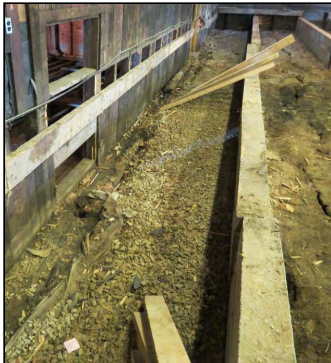
PLATE 8: Granular material between southernmost concrete joist and south wall of the Inshore Fisheries Display Building; facing west; October 22, 2013.
