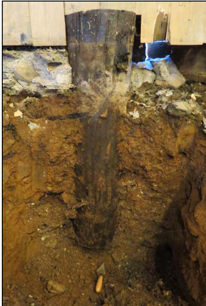
PLATE 13: Test excavation of post along the north wall of the Inshore Fisheries Display Building; facing north; November 5, 2013.
