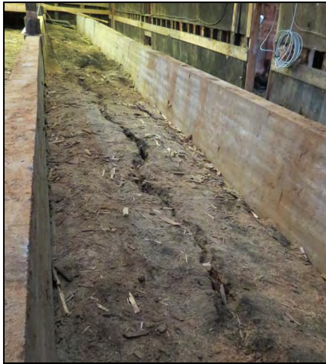
PLATE 9: Cracked and slumping clay fill and concrete joist along southern end of the Inshore Fisheries display Building; facing east; October 22, 2013.
