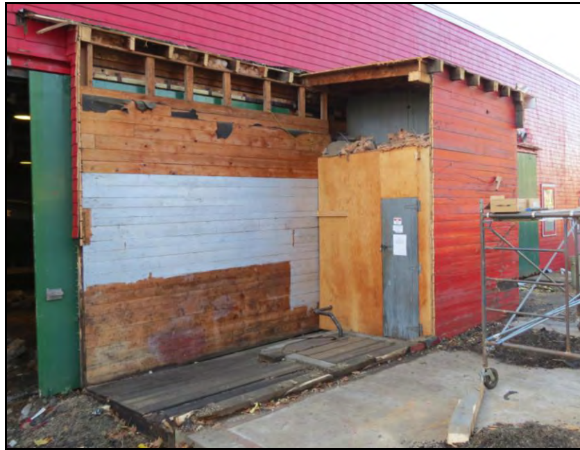
PLATE 26: Mechanical room following the dismantling of the wooden structure; facing southwest; October 25, 2013.
