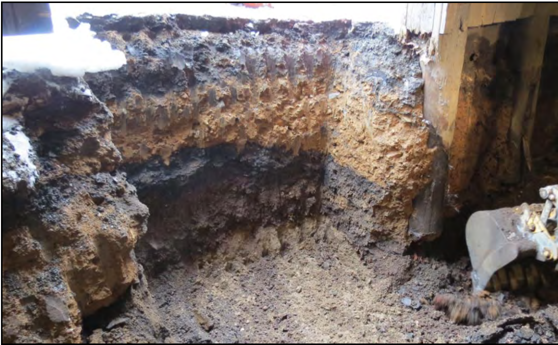
PLATE 20: Oblique view of north profile of excavation pit along north wall of the Inshore Fisheries Display Building; facing northeast; April 2, 2014.
