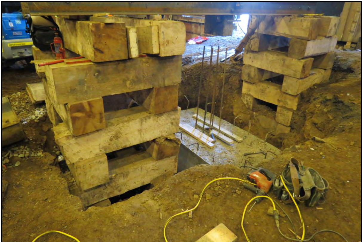
PLATE 16: Concrete piling cap poured in excavation pit between timber supports in north central portion of the Inshore Fisheries Display Building; facing northwest; January 8, 2014.
