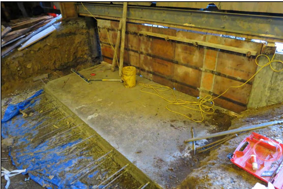
PLATE 21: Concrete slab forming part of the foundation of the FMA mechanical room; facing northwest; January 8, 2014.
