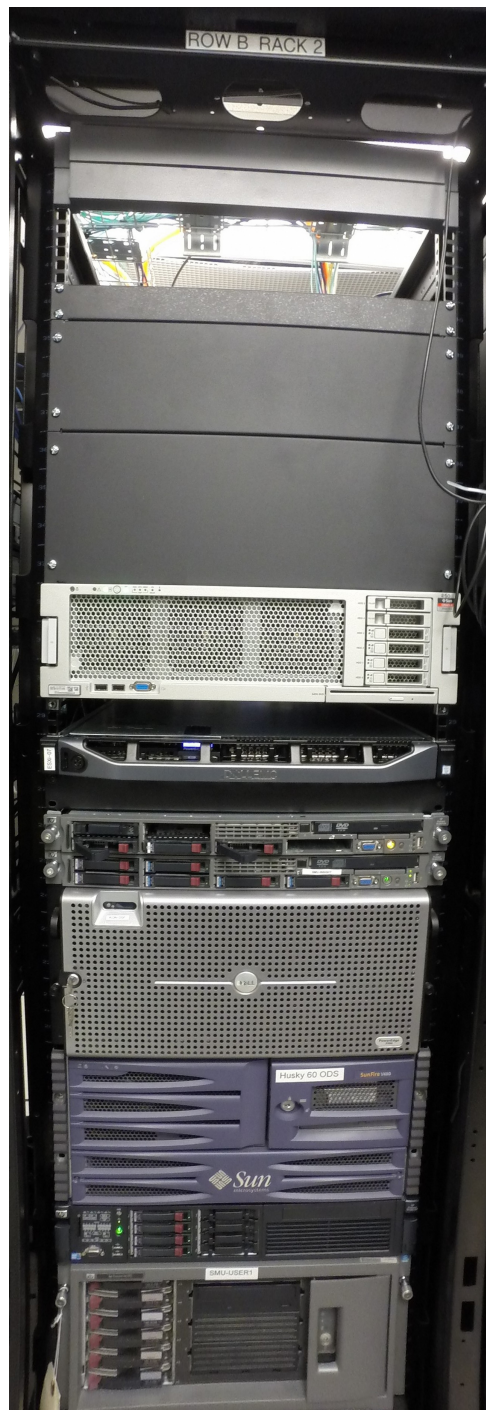
Figure 9: Image of a server rack after undistortion and cropping
