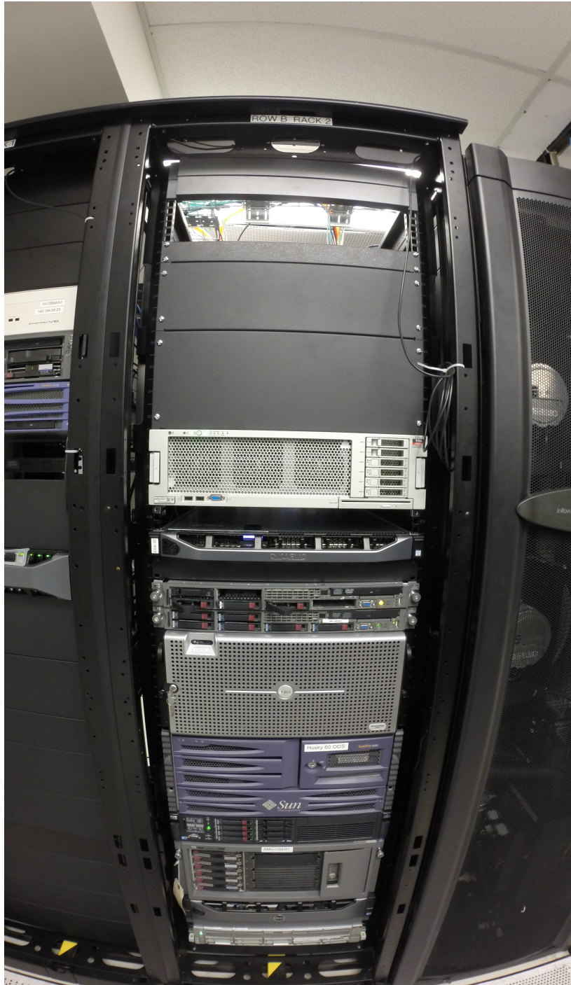
Figure 8: Raw image of a server rack taken with a GoPro 4 camera
