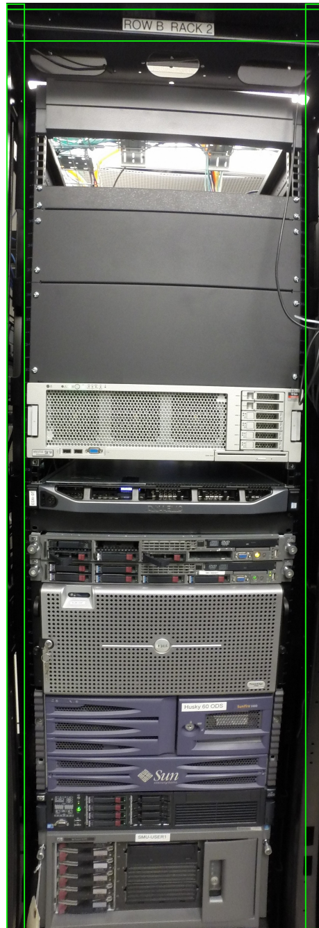
Figure 20: Rack 2, with the perimeter of the rack outlined in green
