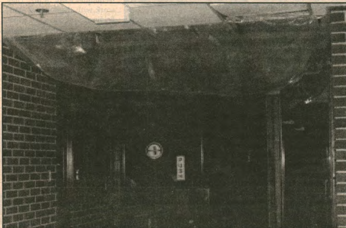
WATER, WATER ALL AROUND. JUST ONE OF THE LOCATIONS WHERE WATER HAS BEEN LEAKING THROUGH FAULTY WALLS AROUND CAMPUS.
