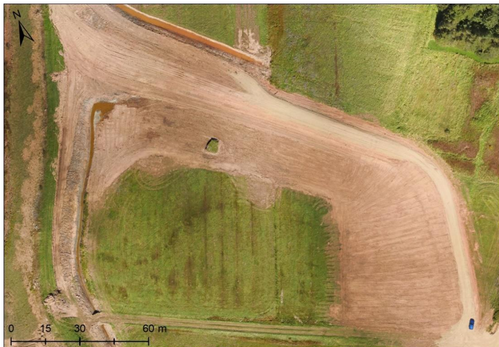
Figure 2.3. Converse restoration site borrow pit excavation prior to site breach. Imagery collected with a DJI Phantom 3 RPAS on September 24, 2018.
