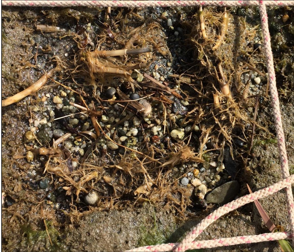
Figure 3.23: Scouring of seed plots at Lawrencetown Lake from high wave energy (1-week post construction)
