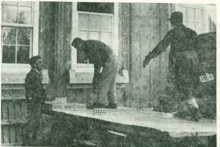
Workmen put finishing touches on University building. Father Brown informs us brick work will be finished before we go to press. Work on the chapel will be completed before Christmas, weather permitting. After Christmas?
