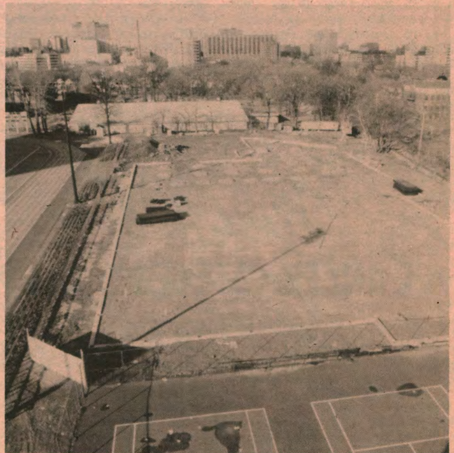
Construction of the new Fitness and Recreation Centre has been delayed slightly due to the weather and the fact the structural steel has not yet been delivered. It's a minimal delay, though, says Guy Noel, Vice-President (Administration), and the contractors still say the project will be completed on time. (Chislett photo)
