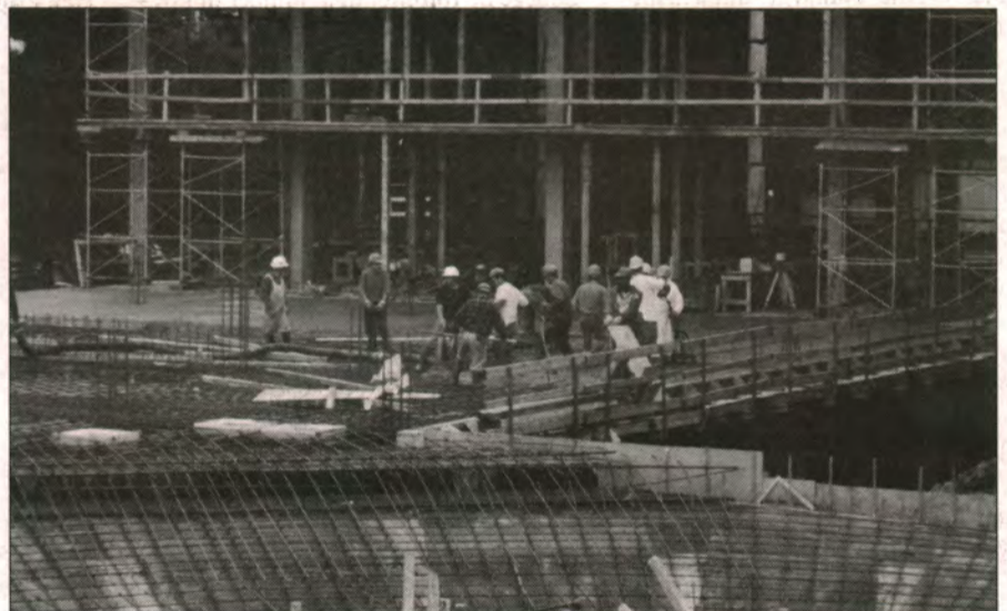
The construction workers grind it out each day to ensure that the University's new school will be open by next summer.
