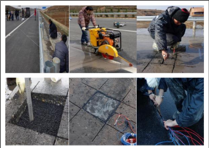
Figure 9. - The installation process of PE tiles on Ma-Zhao highway Zhaotong City, Yunnan Province, China [115].
